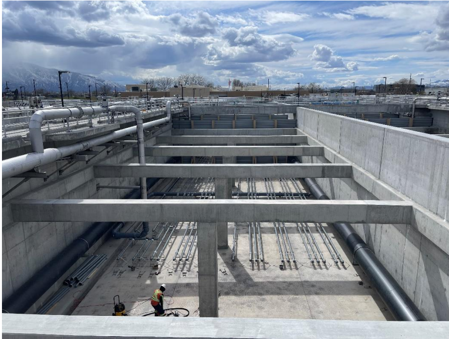
View looking S/E at Train #2 of the Aeration Basin
