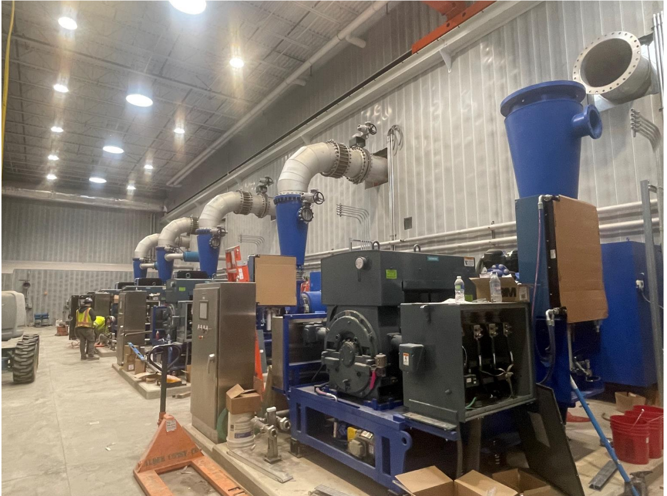
View of the Five Lonestar Blowers in the Blower Room, looking S/W
