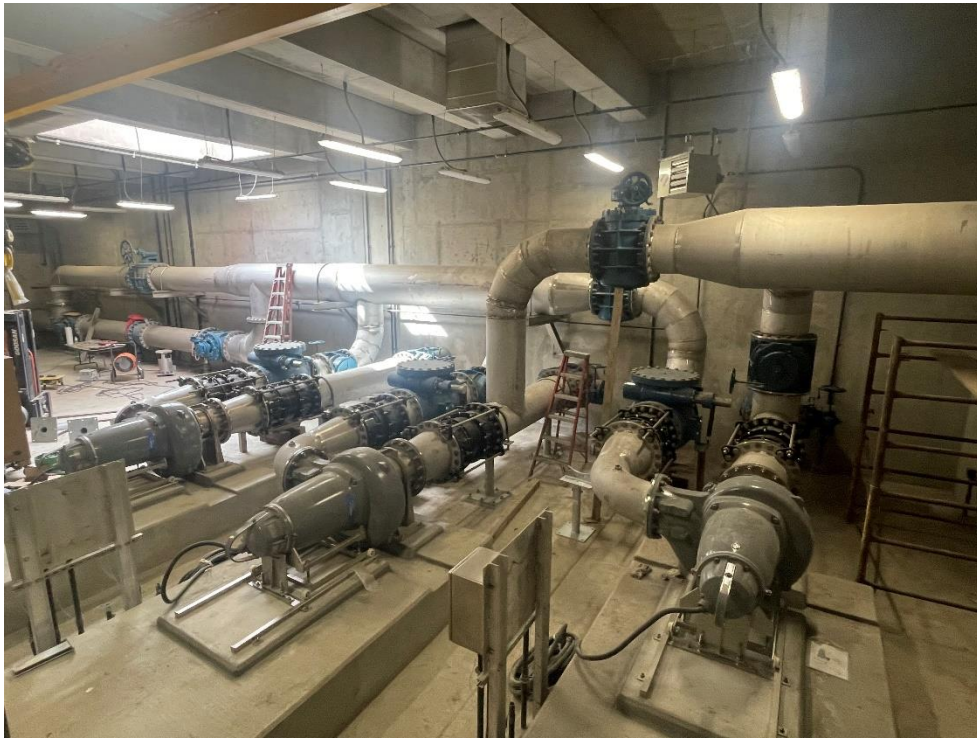
RAS Dry Pit Mechanical Piping, Looking Southwest.
