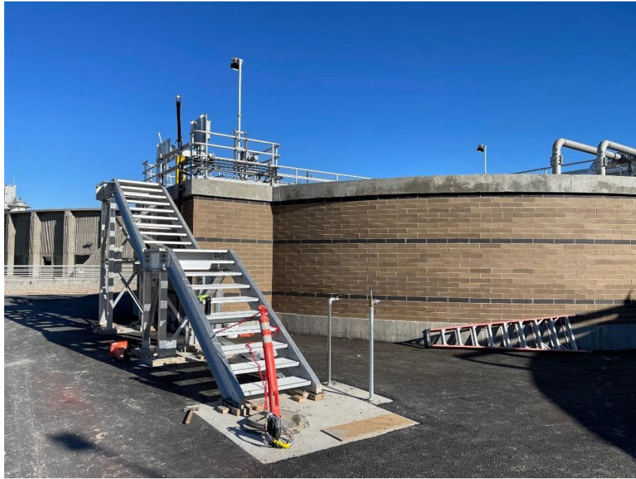
View looking N/E at SSN Reactor #1
